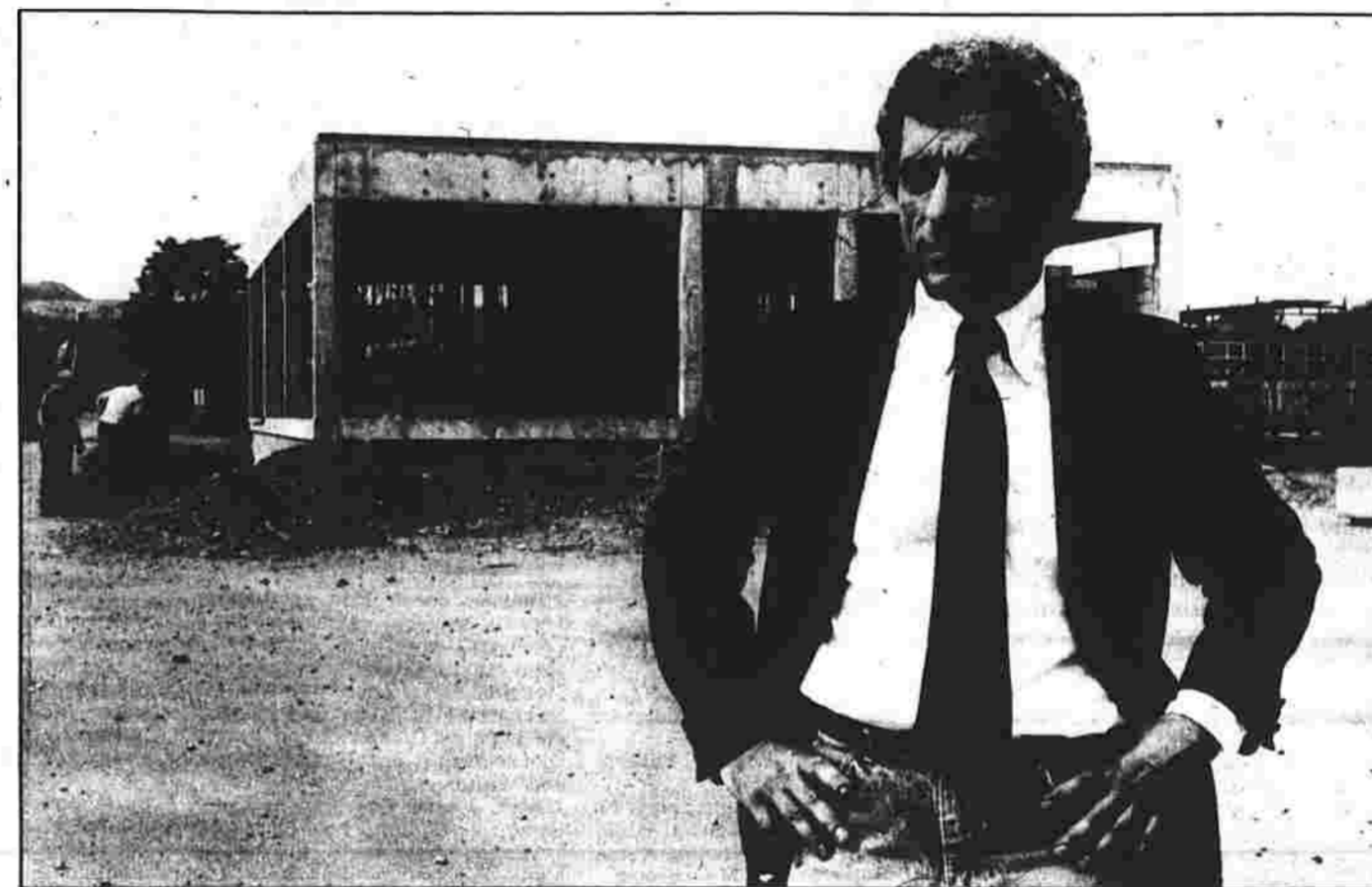
MR. MAYOR — Manchester Mayor Peter P. DiRosa Jr. today stands in front of crews working on the secondary part of the town's sewage treatment
