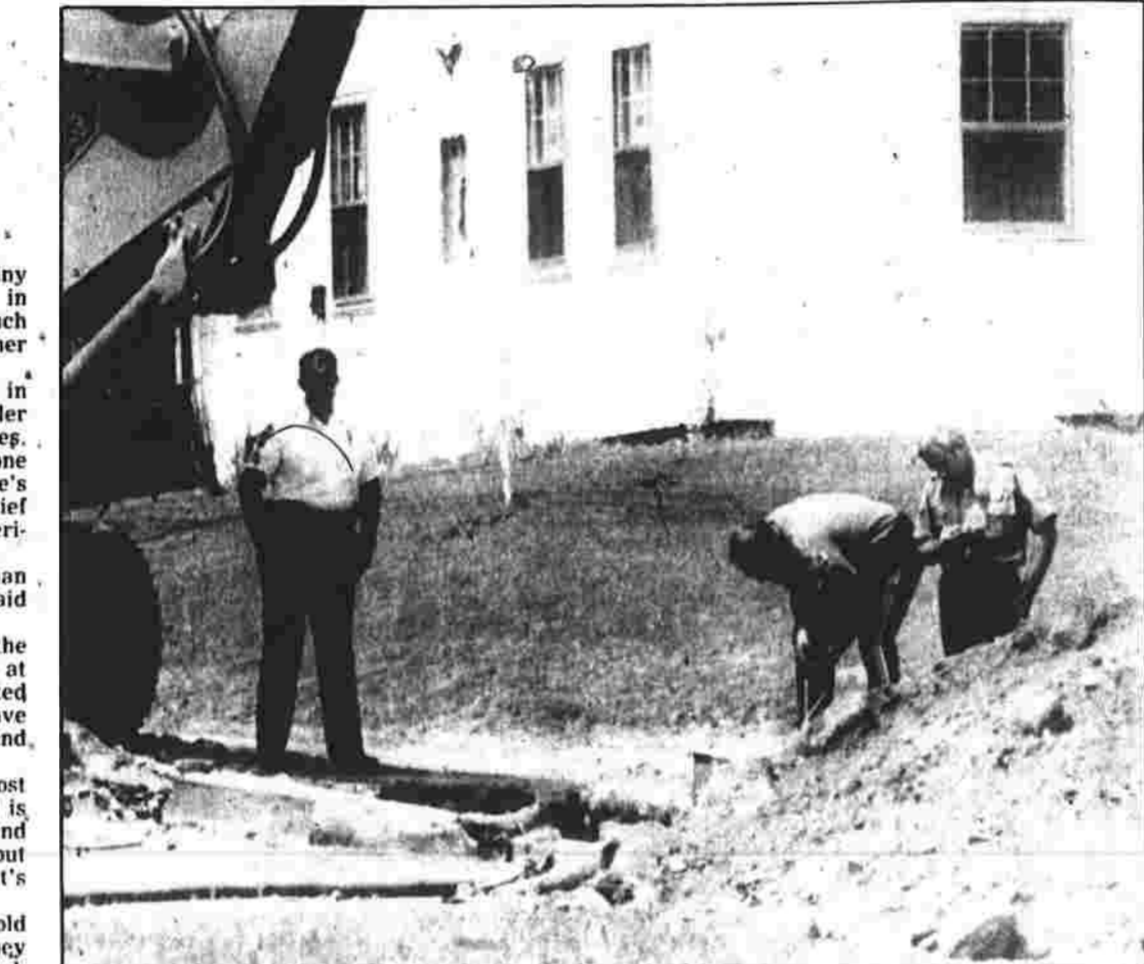
EXPLOSION SITE — Two state police officers peer into a sewer trench in East Granby where an explosion occurred Wednesday morning. The explosion injured two workers and trapped them for 35 minutes.
